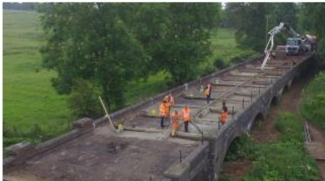
Image above: NLR volunteers restoring Bridge 11, at the northern end of the extension, Summer 2019.
